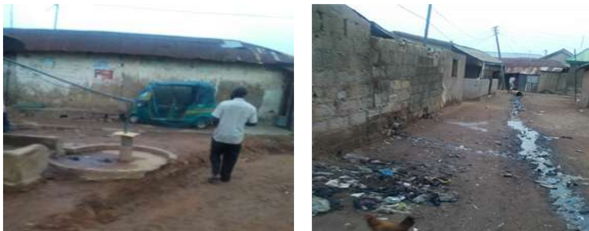
Plate 3a & b: Laterite road works on-going and typical inner street as drainage as well. Source: Field Survey (2017)
